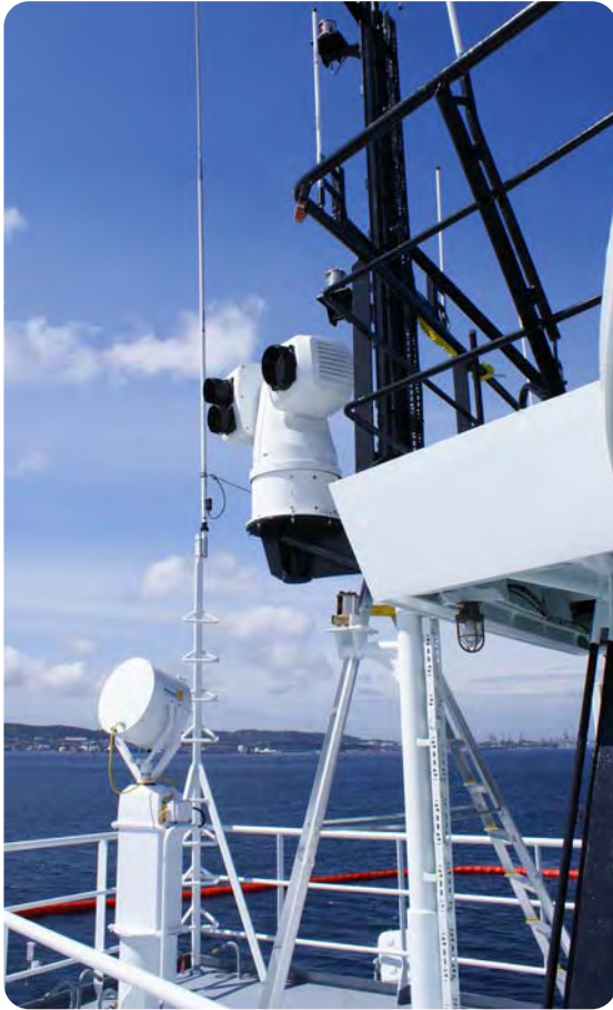
The SECurus system is installed on the supply vessel Volstad Princess owned by Volstad Shipping under contract to StatoilHydro.
